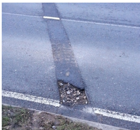
An example of poor & unfinished reinstatement work along a duct trench near Mentmore in 2015.
